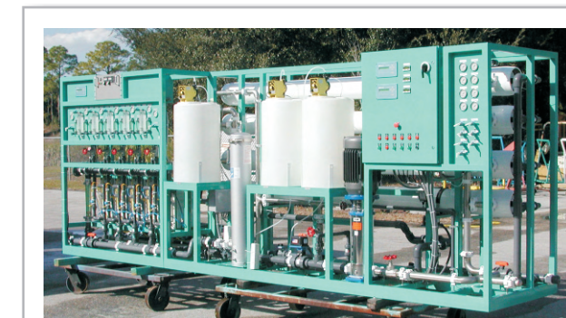
Reverse Osmosis - Electrodionization (EDI) - Chemical Dosing
